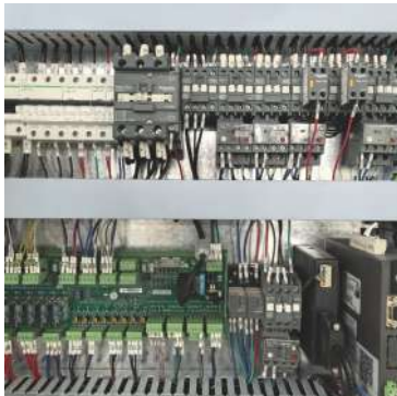
SCHNEIDER brand electric parts
